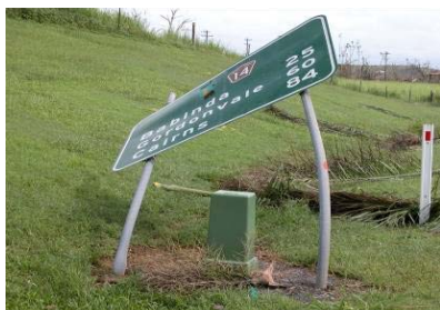
Failed road sign (used to determine local gust wind speeds)
