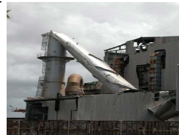
Collapsed chimney stack – Mourilyan sugar mill
