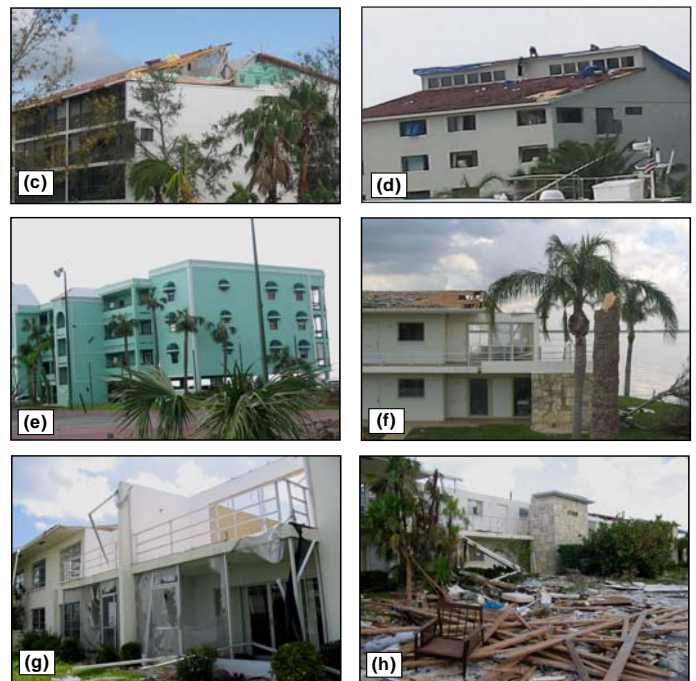
Figure 1 (continued). Comparison of pre- and post storm building conditions in satellite images, along with ground-survey photos. Ground-survey photos demonstrate: (c) partial roof deck failure (combined internal and external pressures); (d) shingles partially removed but deck intact; (e) scoured roof gravel (not visible from ground survey); (f) partial roof structure failure; (g) severe roof structure failure; (h) windborne debris from nearby building deposited on parking lot, roadway, and tennis court.
