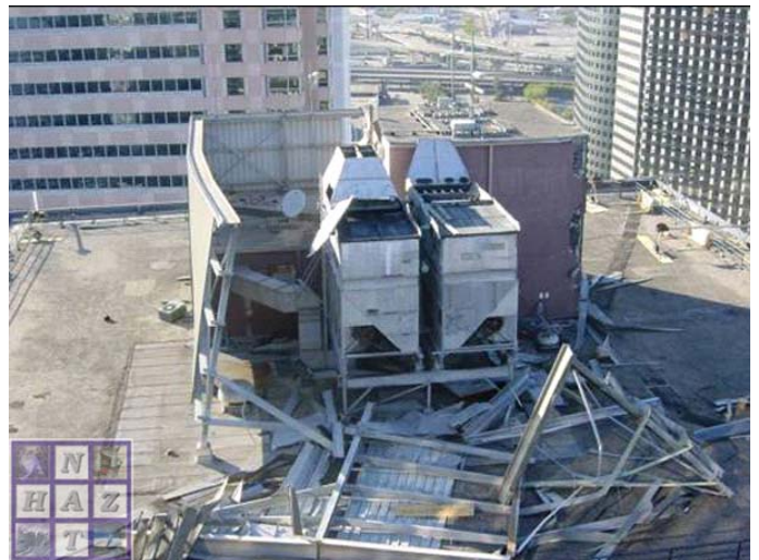
Figure 5 Rooftop penthouse on Amoco Building was nearly destroyed
