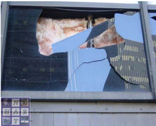
Figure 7 Broken window on north face of Hyatt Regency Hotel, likely caused by missile impact.
