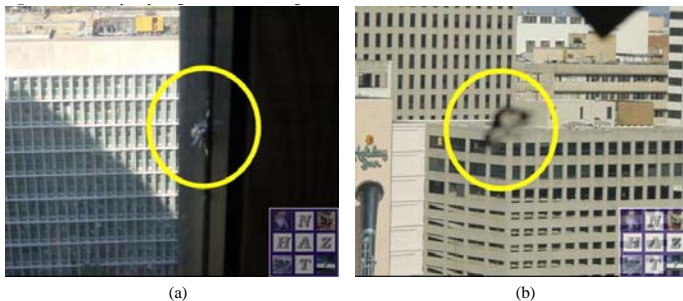
Figure 8 Missile impact pitting on Amoco Building.
