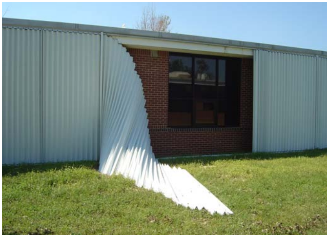
Failed shutters at Sherwood Elementary School in Pensacola (Hurricane Ivan)
