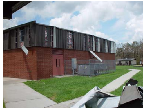
Damaged building at Zolfo Springs Elementary School, courtesy of Hurricane Charley
