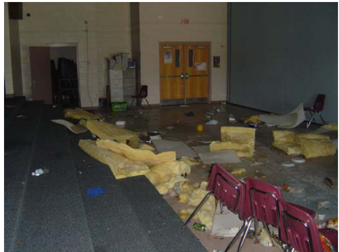
Collapsed ceiling in shelter area at West Florida High School of Advanced Technology, during Ivan
