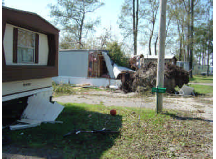
Extensive damage due to falling trees
