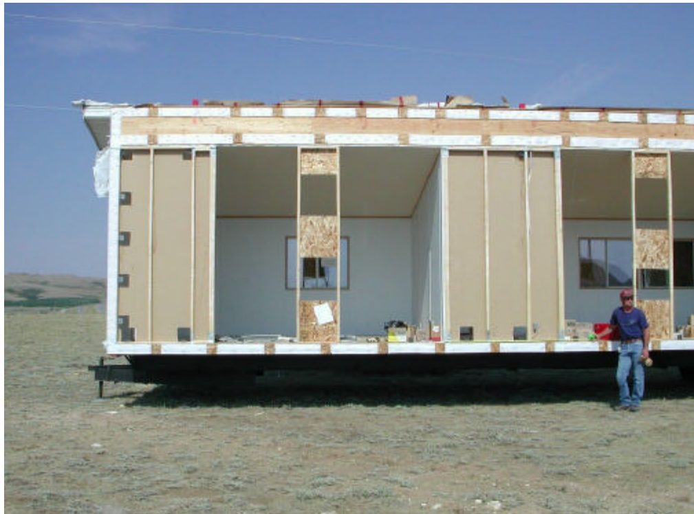
Figure 1. Load cells installed at the marriage line of this double-section test home will provide wind load transfer data
