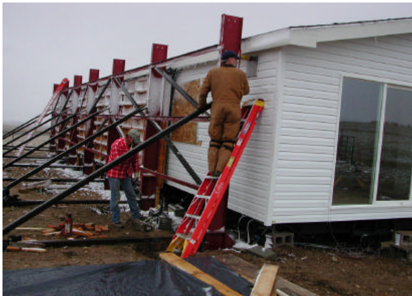
Figure 3. Data from point loads up to 3500 lbf applied just below the eave of the west exterior wall to be compared to FEM results
