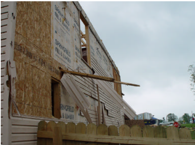
Figure 6 Severe damage to residential structure. Note missile penetrating wall
