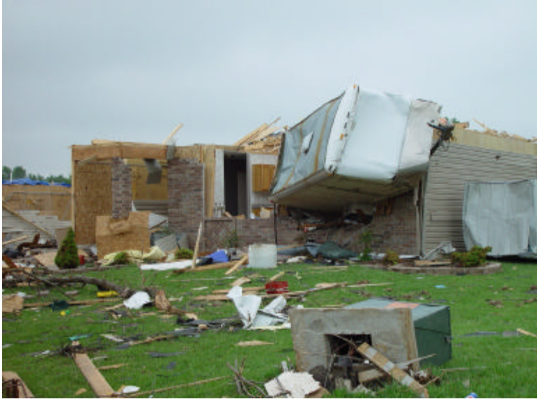
Figure 5 Horse trailer became a missile and struck house. This house lost its roof structure
