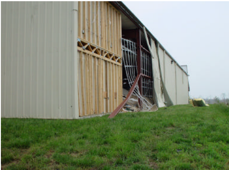
Figure 9 Damage to retail facility
