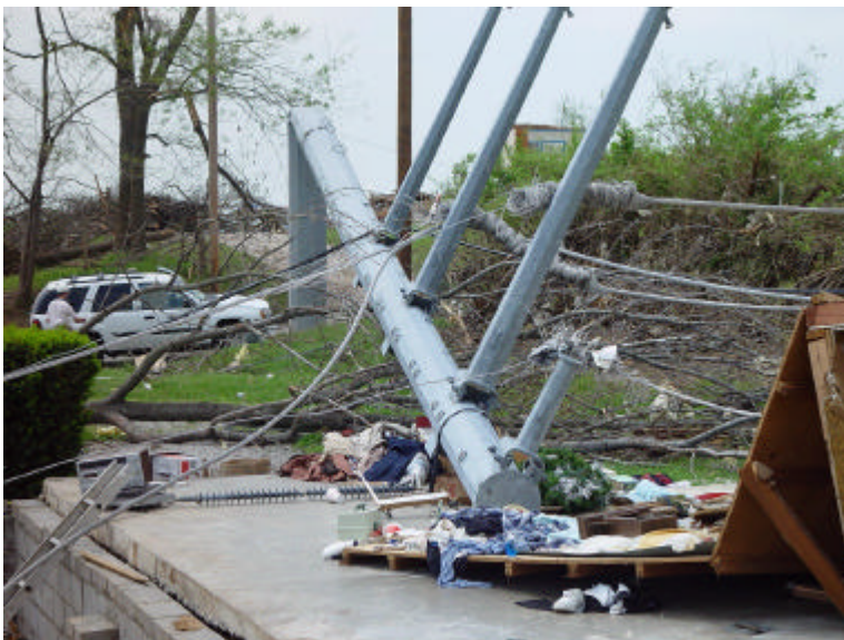
Figure 22 Metal transmission tower struck residence
