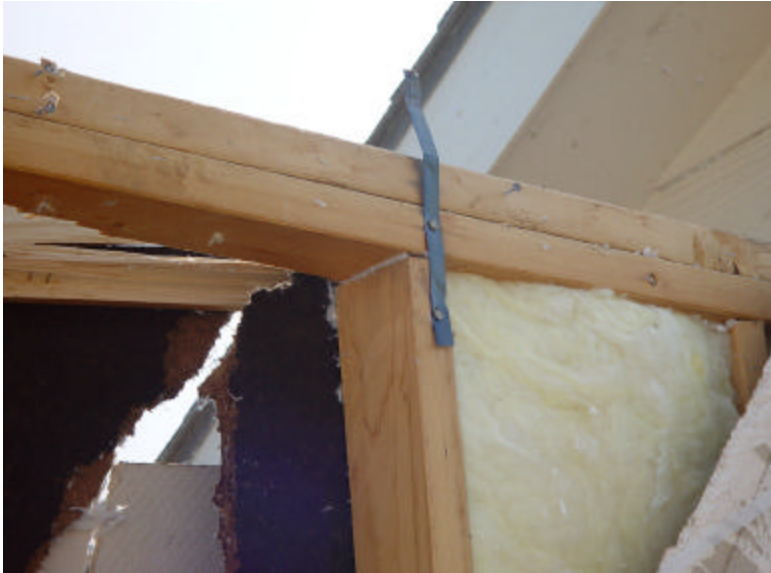
Figure 24 Failure of strap between wall and roof truss
