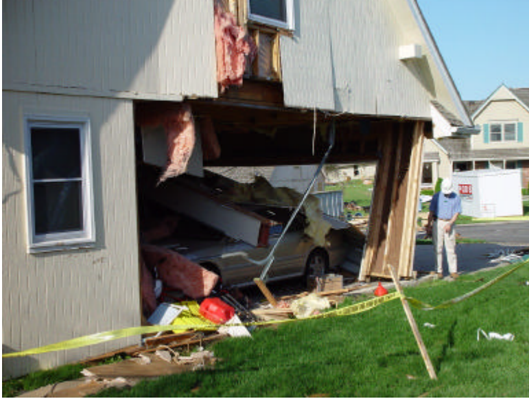
Figure 14 Garage door and wall failure
