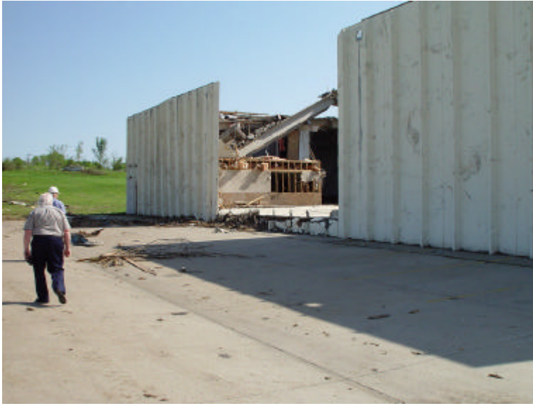
Figure 17 Failure of pre-stressed concrete building
