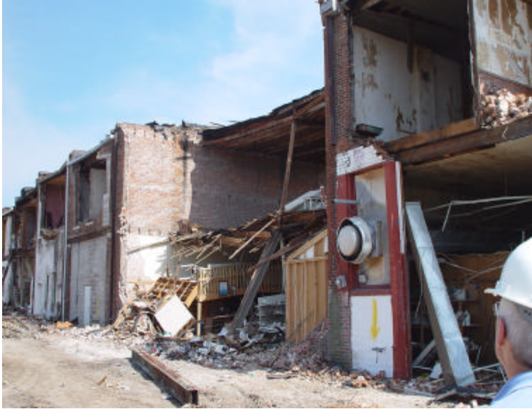
Figure 2 Most of historic business buildings in Pierce City were damaged
