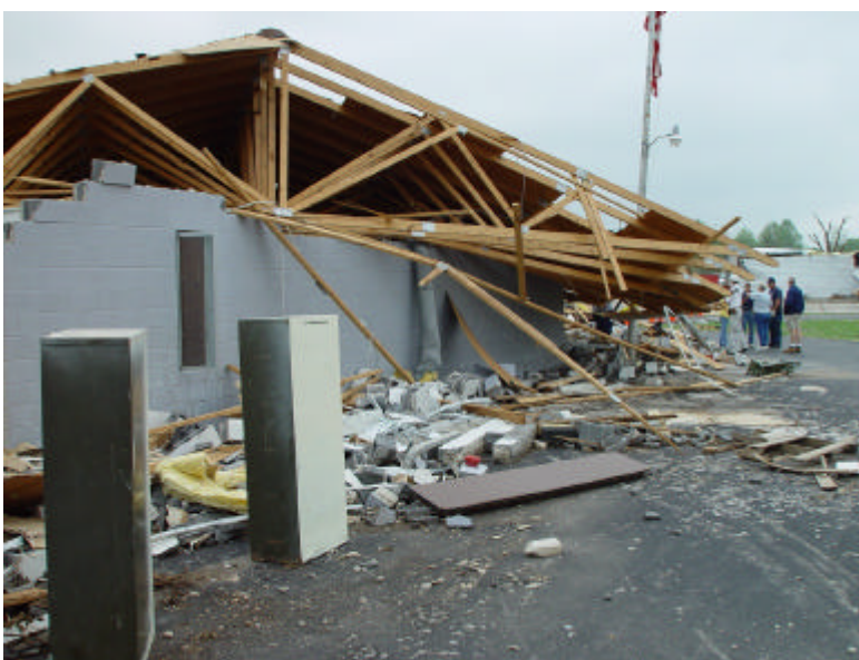
Figure 7 Damaged fire station
