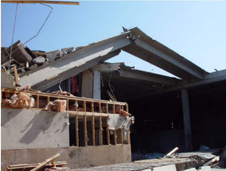
Figure 18 Failure of roof beam due to combined effects of wind uplift and pretension. The beam seats did not provide resistance to wind uplift
