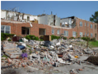
Damaged dormitory (see story on p. 2)
