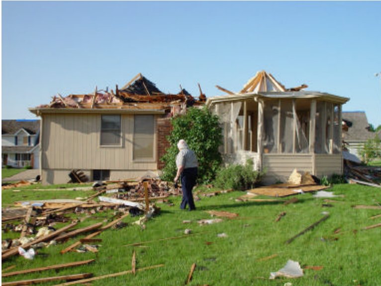
Figure 15 Collapse of brick chimney and loss of roof structure
