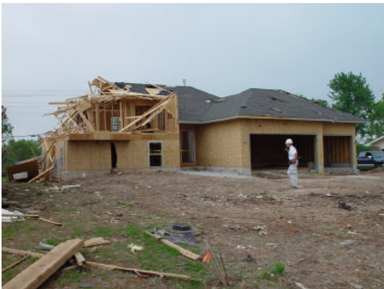
Figure 4 Damage to house under construction
