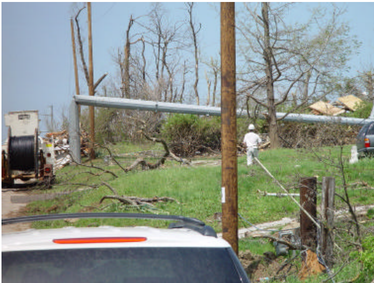
Figure 21 Collapse of metal transmission tower
