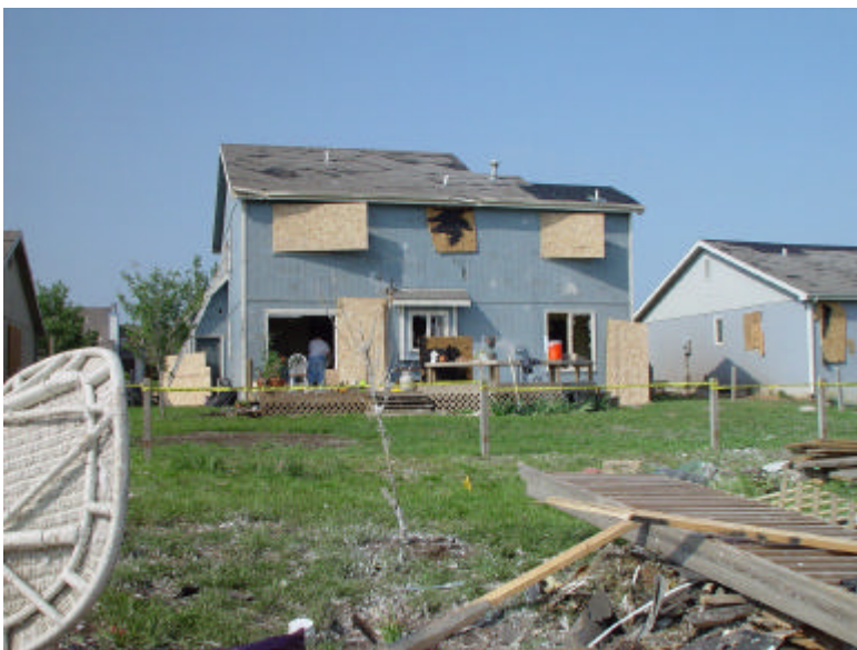
Figure 25 Damage to residence caused by debris from adjacent apartment complex
