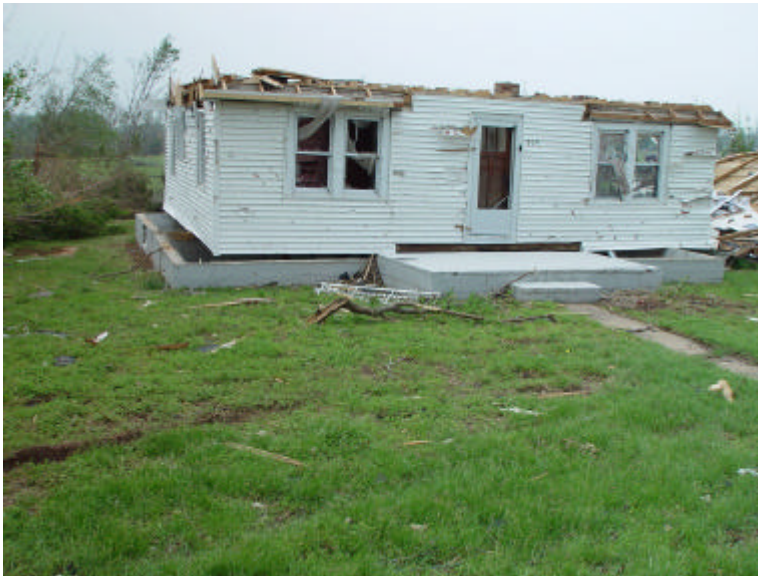
Figure 12 House shifted off its foundation and lost its roof structure
