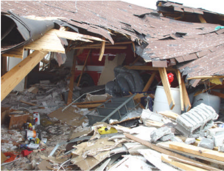
Figure 8 Emergency/fire rescue vehicles were trapped inside the fire station
