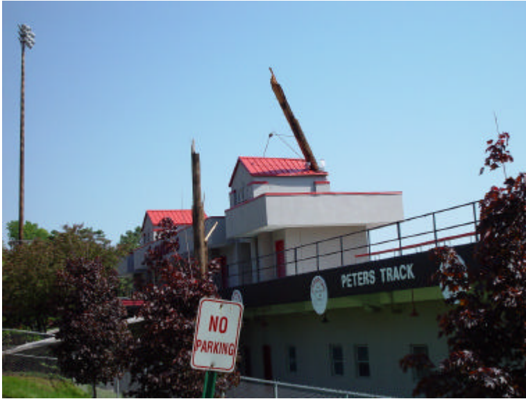
Figure 20 Failure of stadium light standards at William Jewell College
