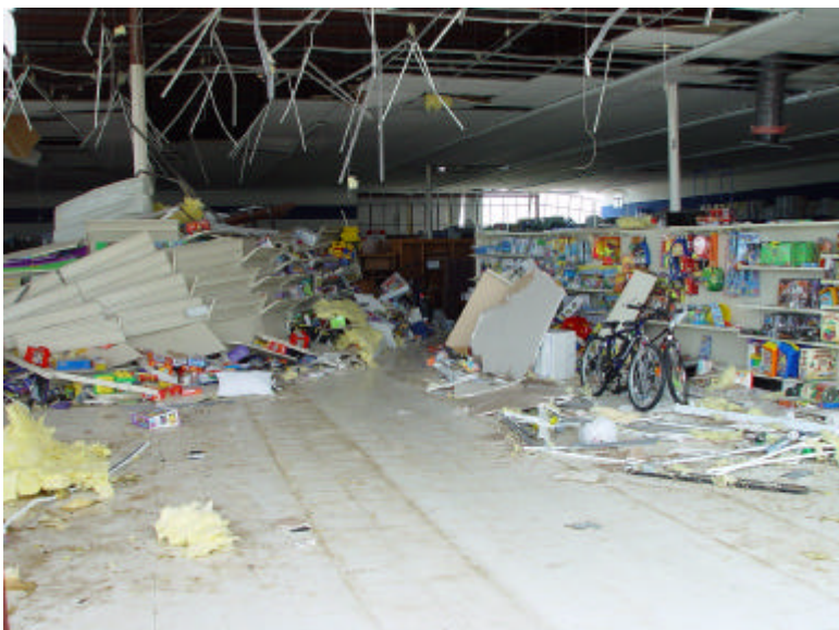
Figure 10 Damage of interior of retail facility
