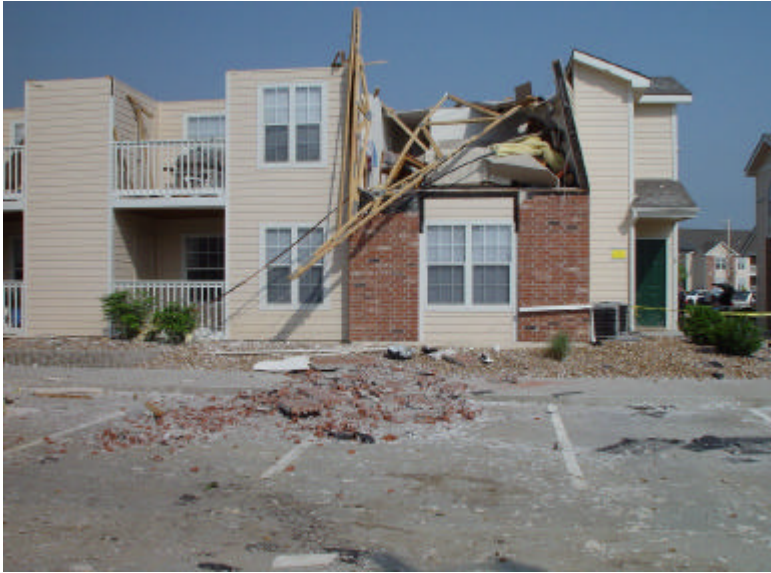
Figure 23 Failure of apartment complex in Lawrence, KS
