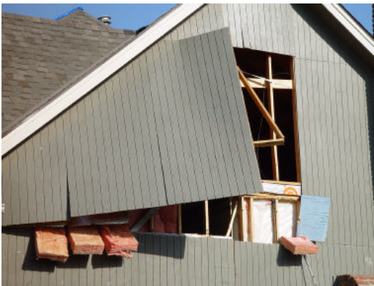
Figure 13 Loss of wall sheathing due to wind suction
