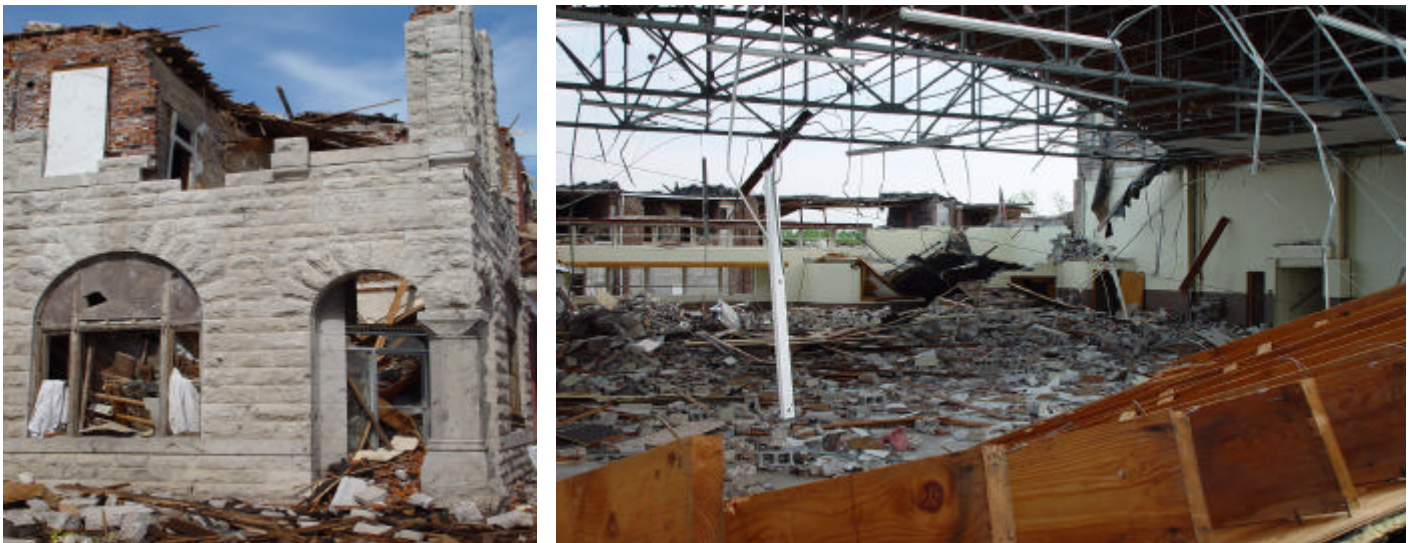
Figure 1 Exterior and interior of the National Guard armory in Pierce City, where people sought shelter. One fatality was reported
