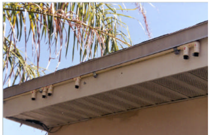
Fig. 4. Sensor Wiring and Outlets
